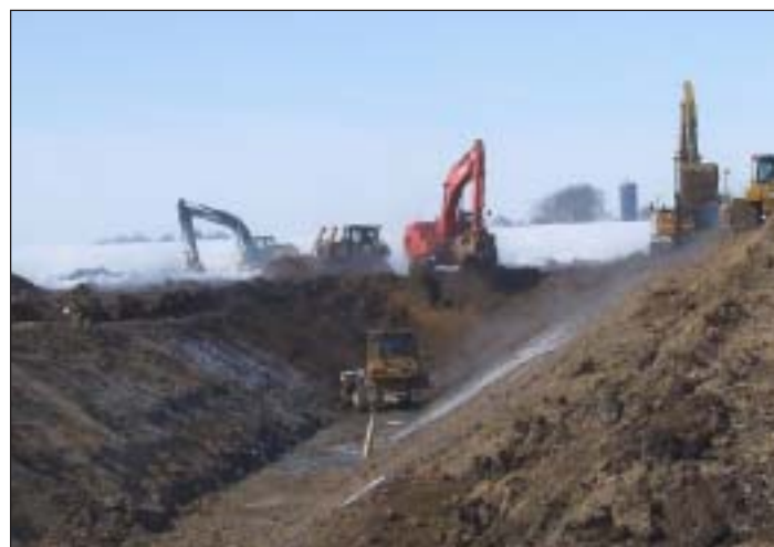
The contractor Redings Gravel and Excavating of Algona defies an ugly winter and works on Drainage District 65, Pocahontas County,
